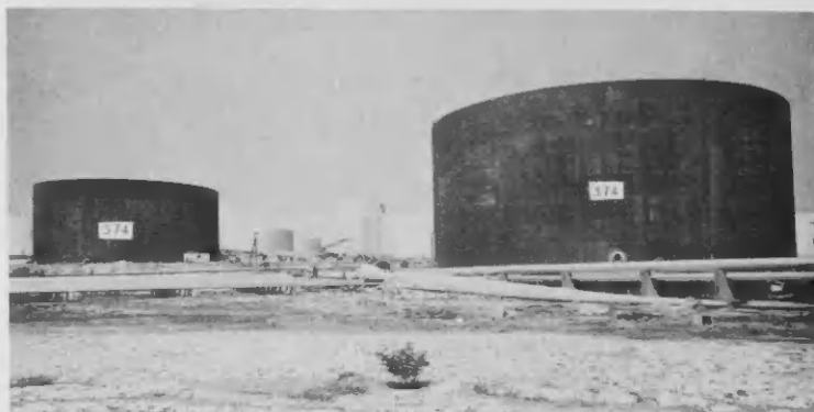
New Kero-Jet Fuel tanks. (Tankinan nobo pa Kero-Jet Fuels).
